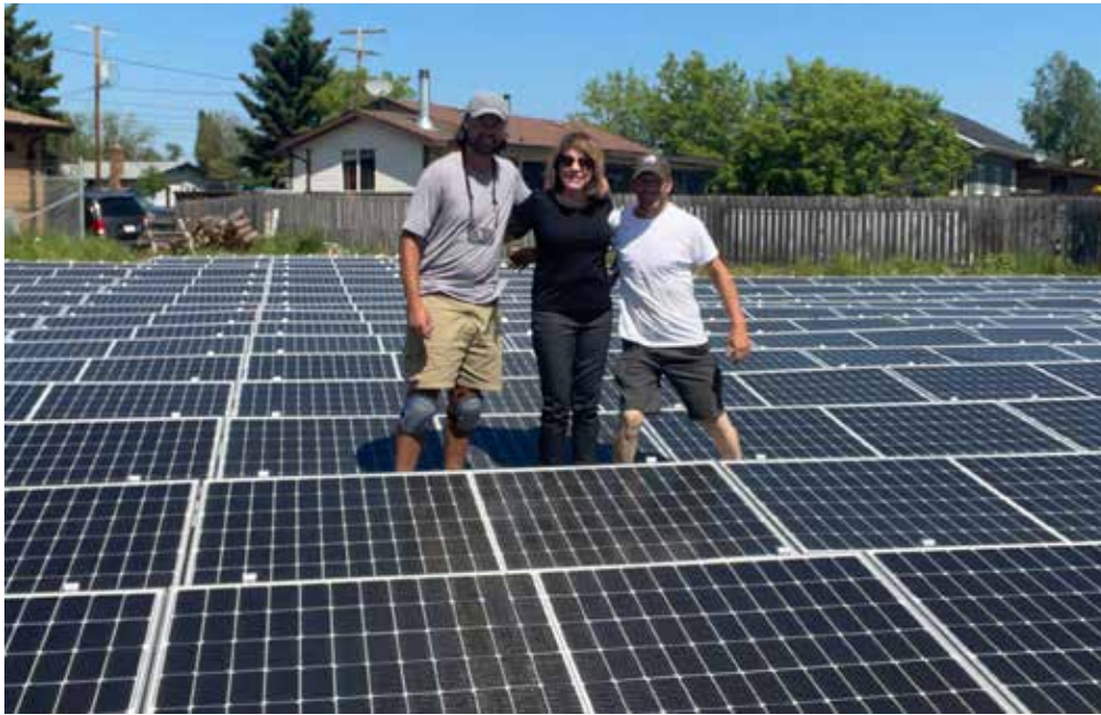
David Isaac, Brenda Green, and Clay Whitney at the solar panels used to power the adjacent greenhouse. (Photo from Brenda Green)
